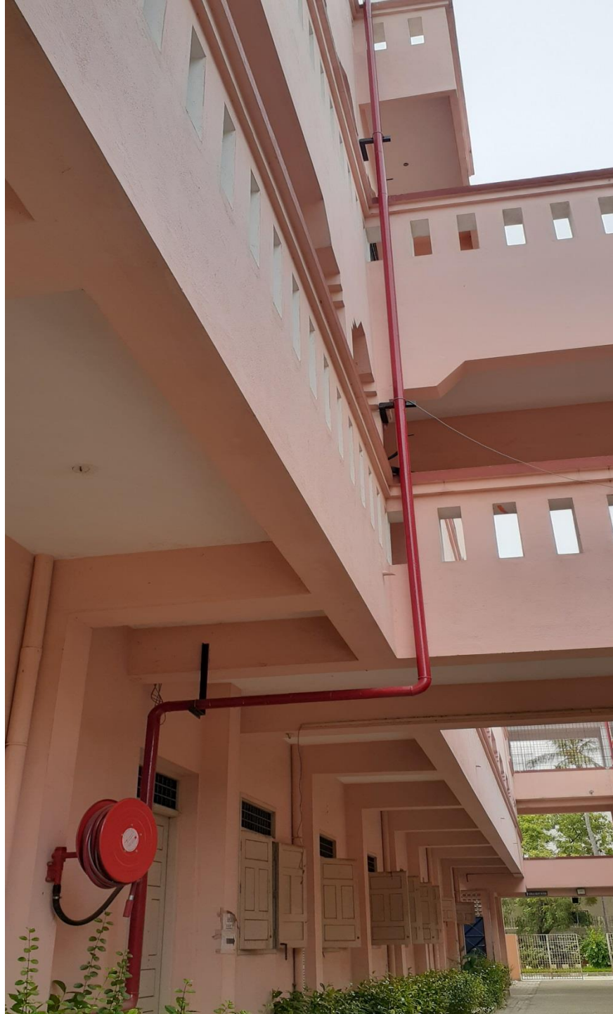
Fire hose in the building
