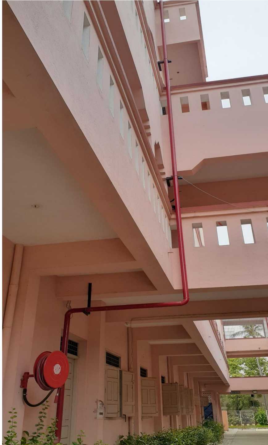
Fire hose in the building
